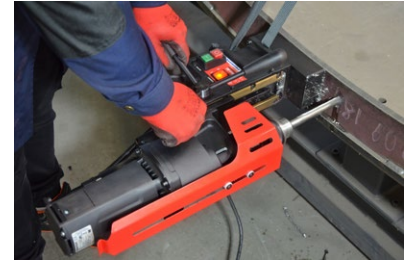
Out of position drilling
